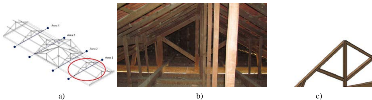
Figure 5: Timber roof truss: a) location on the roof; b) view; c) structure draw
